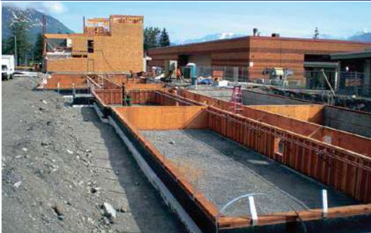
The foundation and site are prepared in Seward while the modules are being manufactured.
