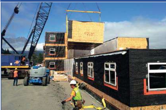
Workers set the modules in place. The project team saved $6 million to $8 million in construction costs and about nine months by using pre-manufactured modular units.
